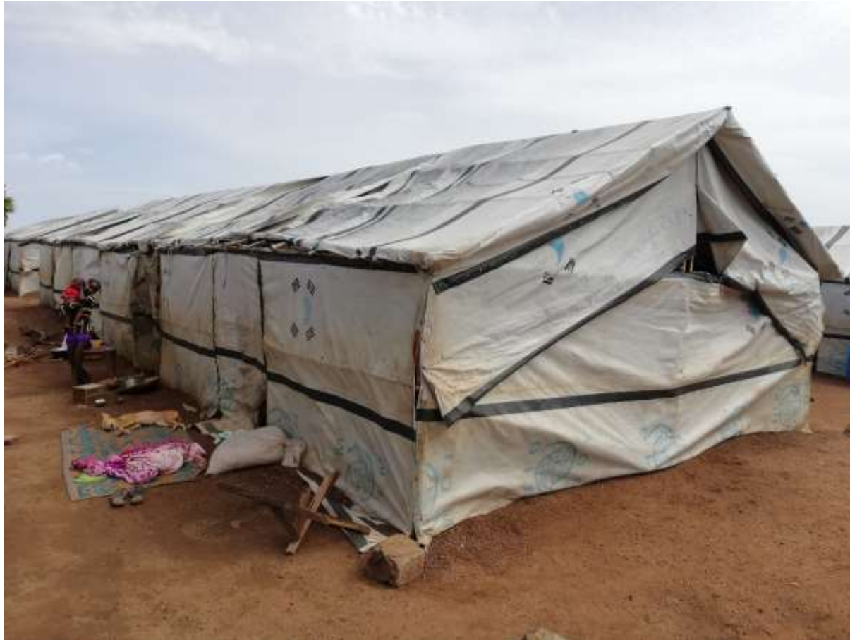
Photo: one of the many damaged communal shelter in Hai masna collective site that requires repair
