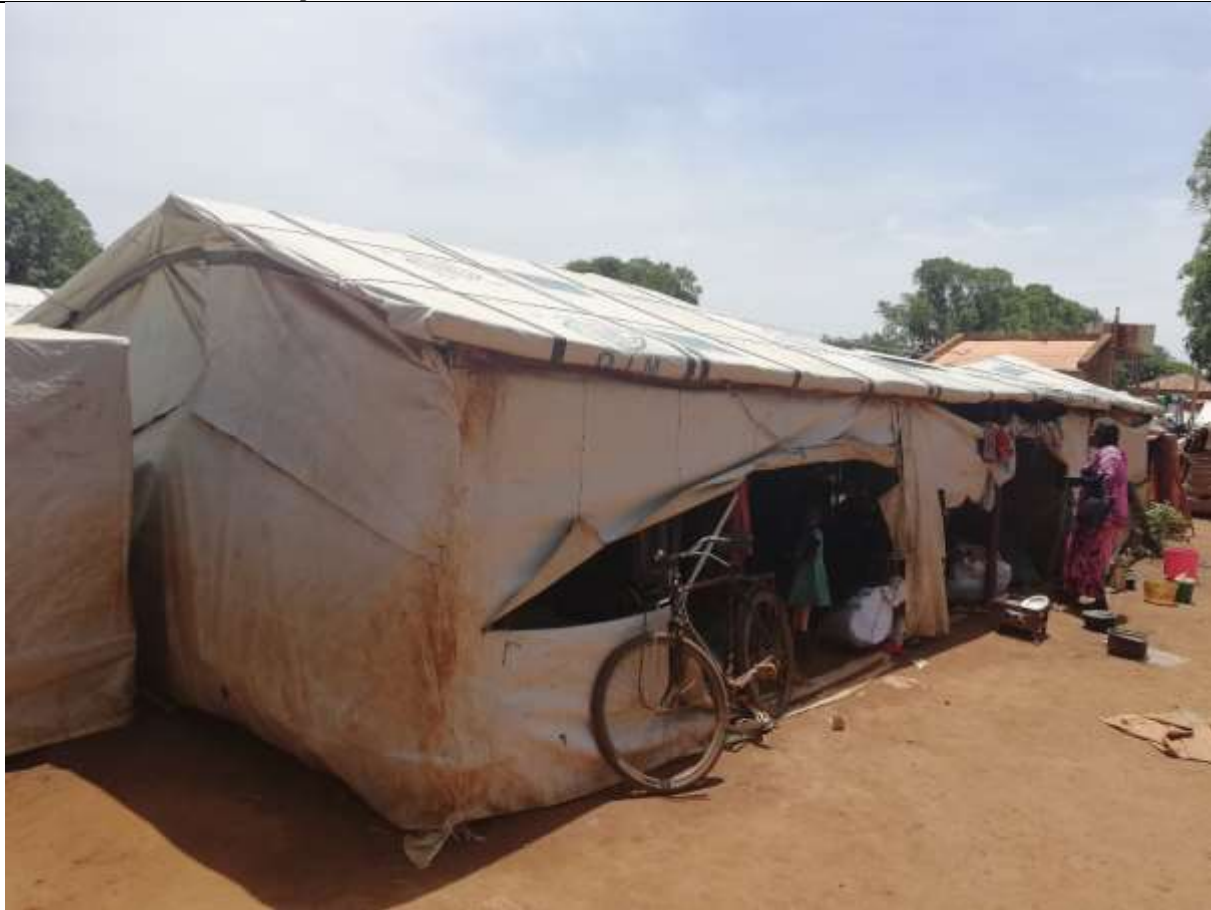
Photo: Damaged communal shelter in Cathedral collective site
